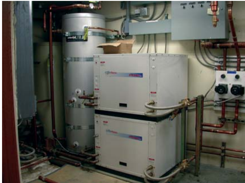
Shown is a typical water-to-water heat pump installation for a radiant floor system. The hot water heater to the left is used as a buffer tank for the radiant floor system.
