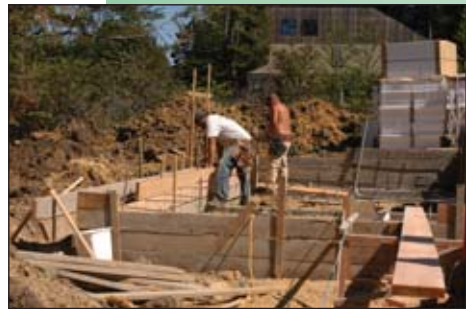
Left: Boat Garage Forms, Underslab Infrastructure, Amvic ICF Wine Cellar, Right: Stormtech Infiltration Chamber
