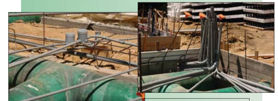
Clockwise: Electrical Conduit Home Theatre, Electrical Conduit Central Control, Amvic ICF Underground Wine Cellar, EnergyEdge/Uponor
